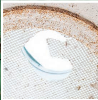
One of John's plastic dome skylights from the inside: hail stones crashed right through. ▲
